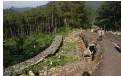
a. Landslide Type Creep at Road (UTM 49M X: 357406 Y: 9193567)
