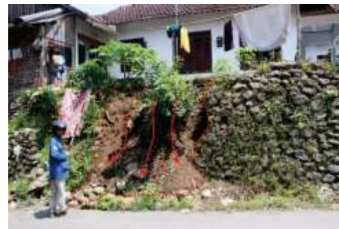
e. Landslide Type Slump at Community Settlement (UTM 49M X: 357406 Y: 9193567)
